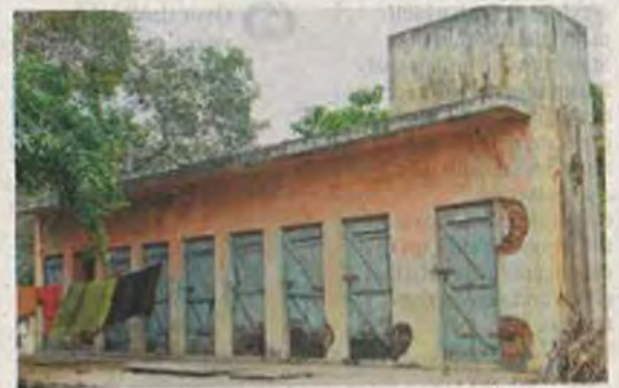
Sorry state: Public toilets at Ayyanar Koil, Thengaithittu, are badly maintained. • T.SINGARAVELOU
